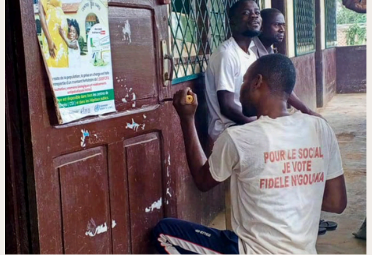
We installed locks to secure the doors at the Bambama Integrated Health Center.
